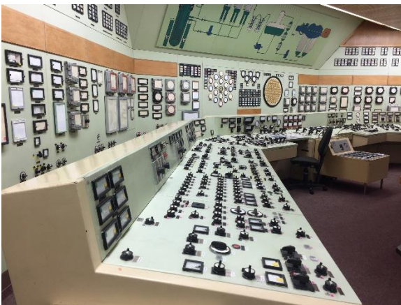
Inside Rheinsberg nuclear power plant. © Jessica Lee. All rights reserved.
